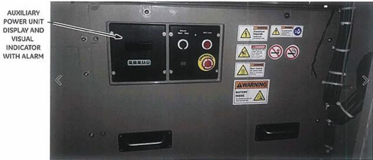
Auxiliary Power Unit
